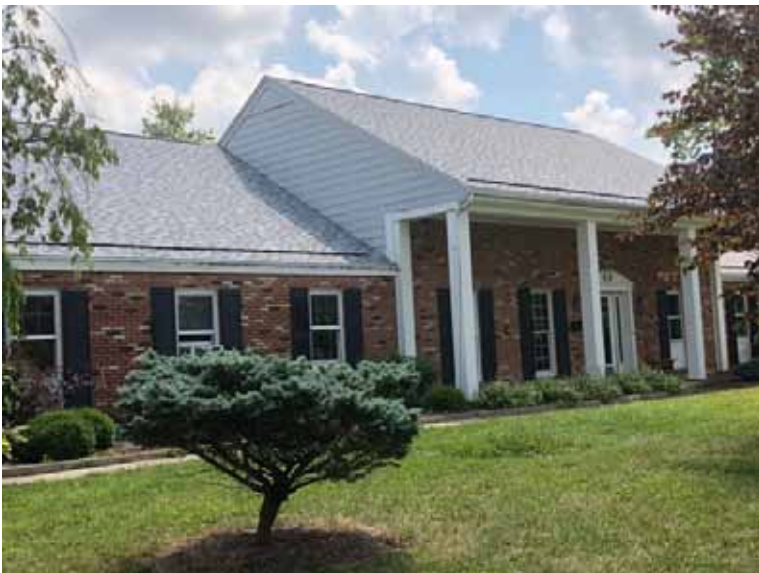
Anonymous Donor with Hamilton Community Foundation Provides a new roof & gutters for Welcome House
